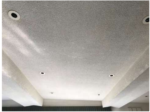
38. View of popcorn ceiling.
