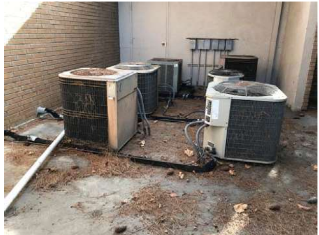
12. View of HVAC units.
