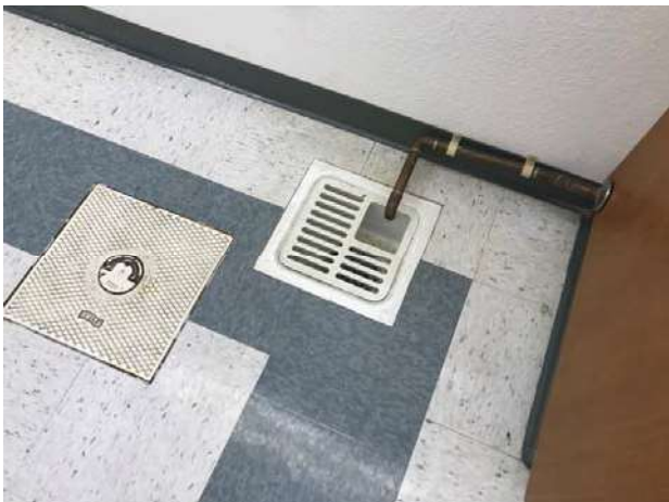
29. View of a floor drain. In the Main Office Building.
