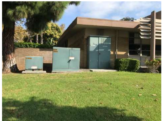
2. View of pad-mounted transformers.
