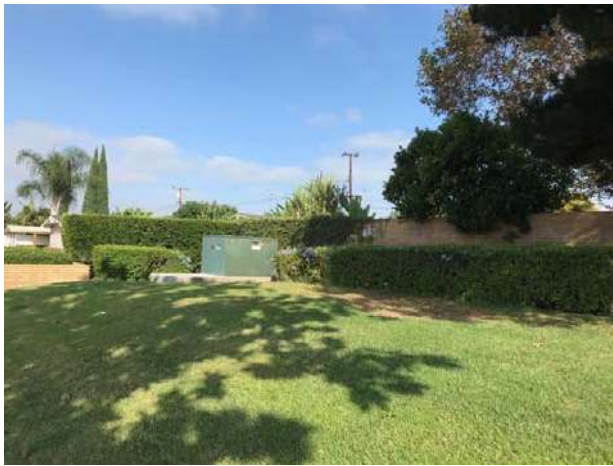
3. View of an additional pad-mounted transformer.
