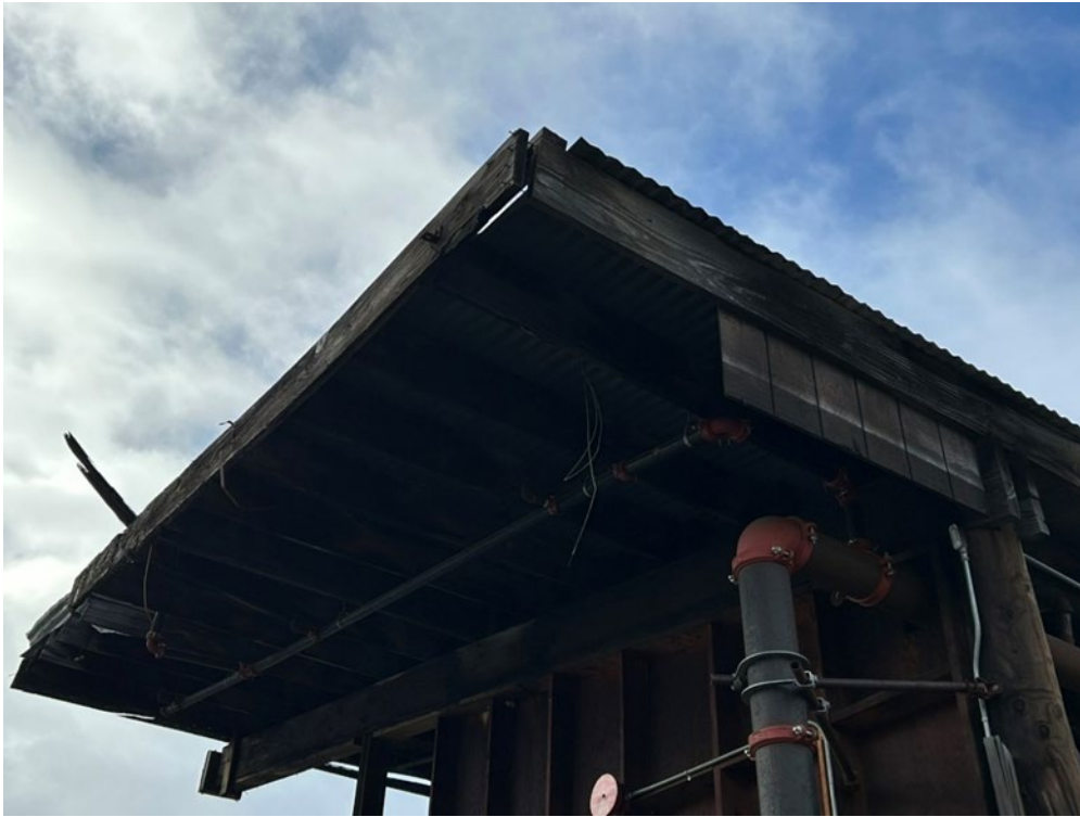
Photograph 61: View of eaves and modern improvements near center of structure, facing southwest.
