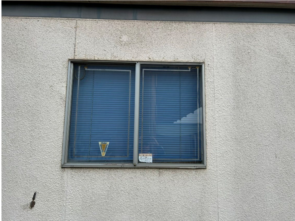
Photograph 25: View of second aluminum double pane window on west elevation, facing east.
