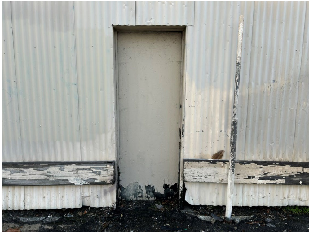
Photograph 34: View of door on north elevation of structure at 301 E. Santa Ana Street, facing south.
