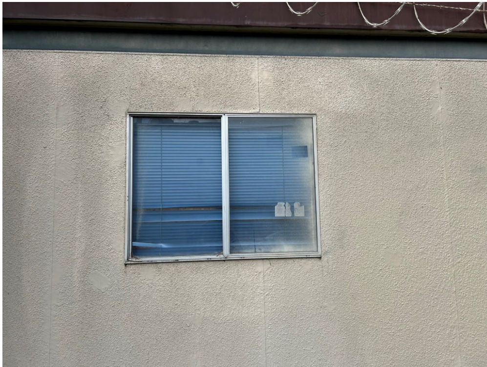
Photograph 29: View of double pane window on east elevation of building, facing west
