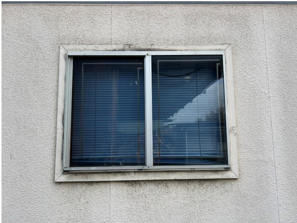
Photograph 26: View of third aluminum double pane window on west elevation, facing east.
