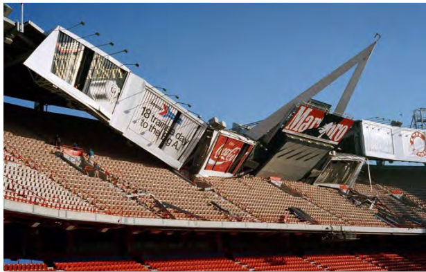
Damage to Anaheim Stadium after the Northridge earthquakes and aftershocks. Image from: https://www.reddit.com/r/angelsbaseball/comments/8gb0z1/remember_the_northridge_earthquake_and_what_it_did_to/
