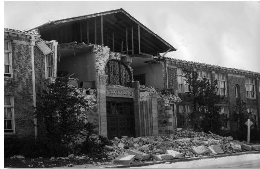
Seismic shaking primarily affects unreinforced masonry buildings, as seen here with this Long Beach middle school damaged by the 1933 Long Beach earthquake. Image from Los Angeles Times.
