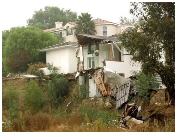
Structural Damage from 2005 Anaheim Hills Landslide Source: OC Register, 2006
