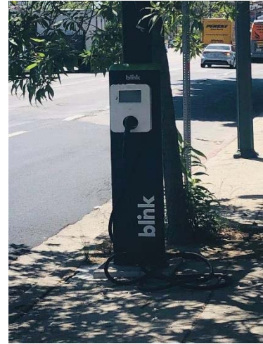
Figure 3. Sample Curbside EVCS
