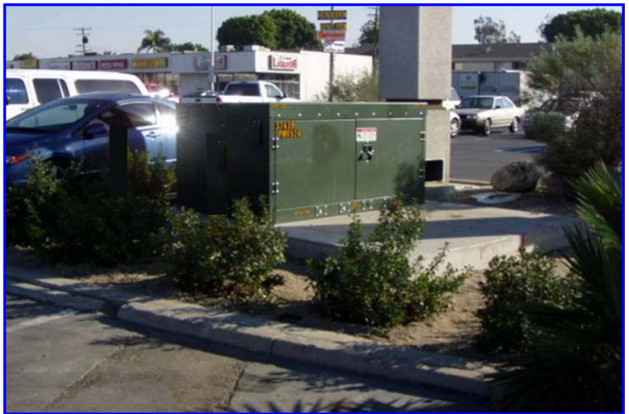
Picture of pad mounted switch. Screening is installed outside easement/clearance area.
