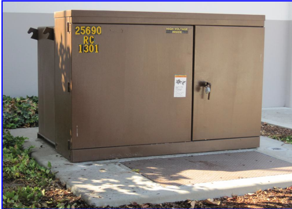
Pad mounted transformer painted to match surrounding environment.
