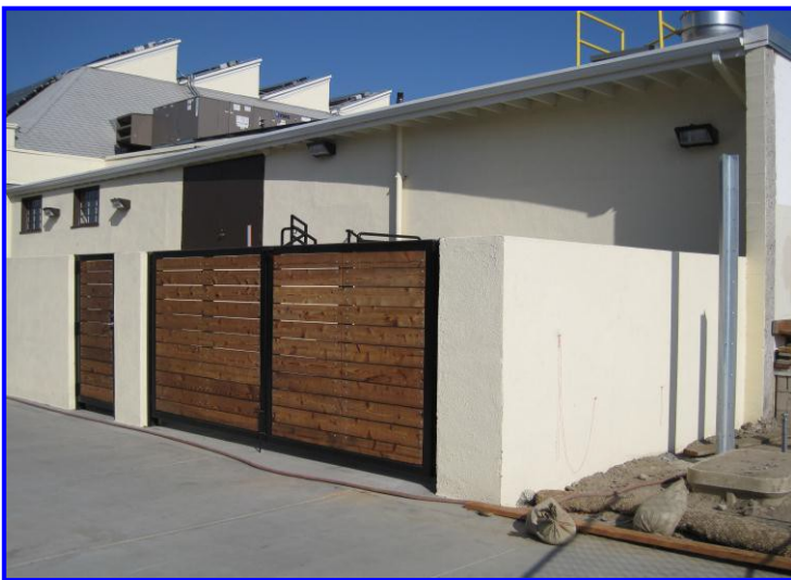
Wall and gate used to screen transformer. See picture to the right.
