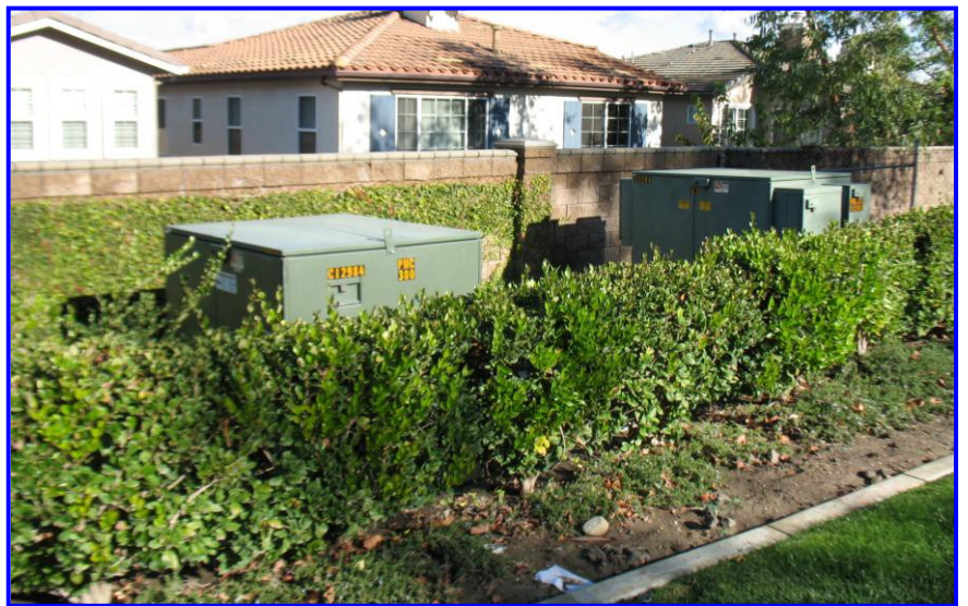
Picture of pad mounted switches. Screening is installed outside easement/clearance area.
