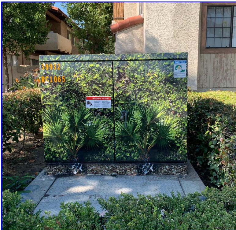
Pad-mounted transformer with graffiti-resistant vinyl wrap to blend in with surrounding shrubs.
