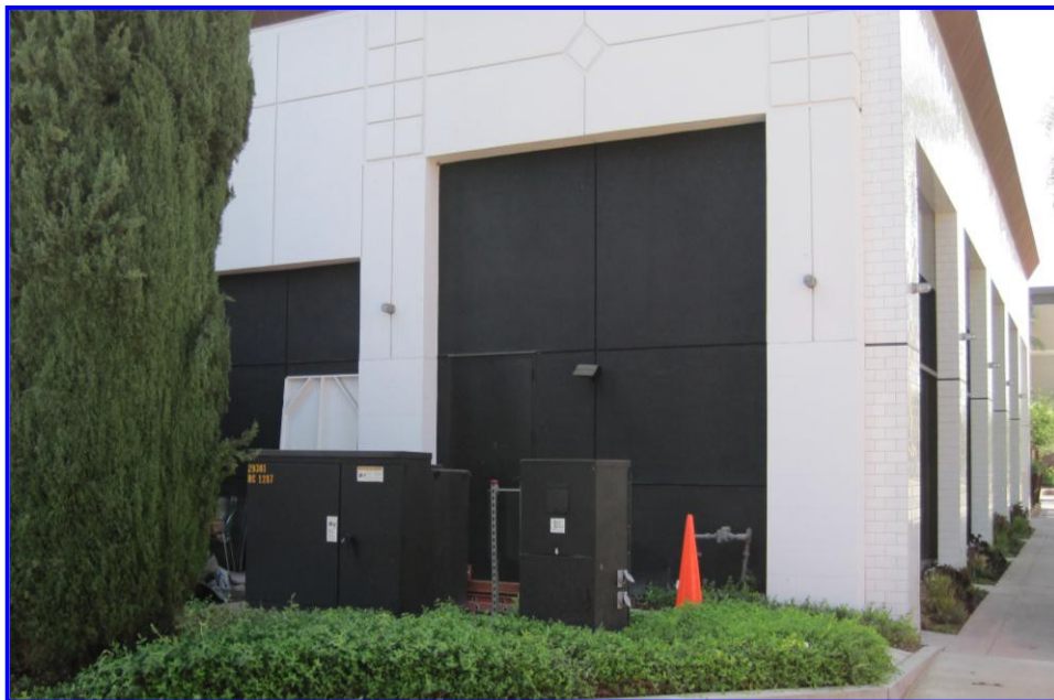
Pad mounted equipment painted to blend with surrounding environment.
