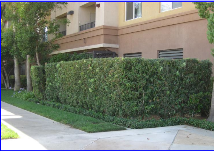
Hedge used to screen transformer. See picture to the right.
