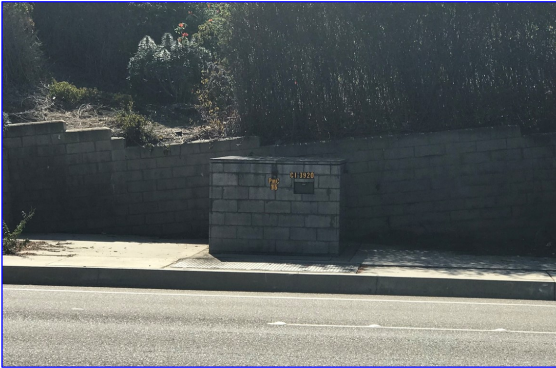
Pad-mounted switch with graffiti-resistant vinyl wrap to blend in with block wall.
